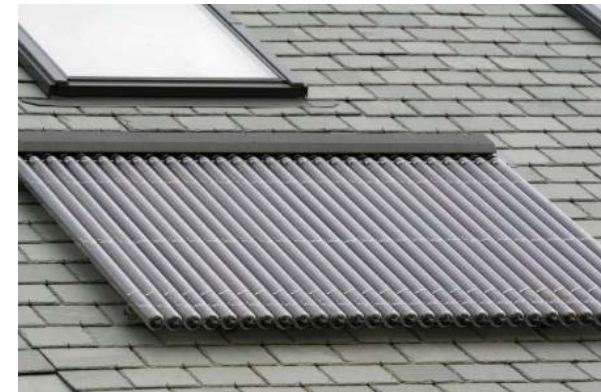
Evacuated Tube Collectors
